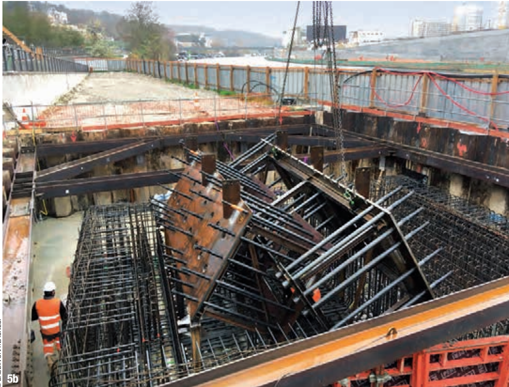
© BAUDIN CHÂTEAINEUF 5b
