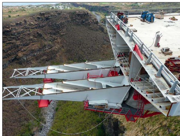
Photo 20 Sabots sur passerelle support Shoes on walkway platform
