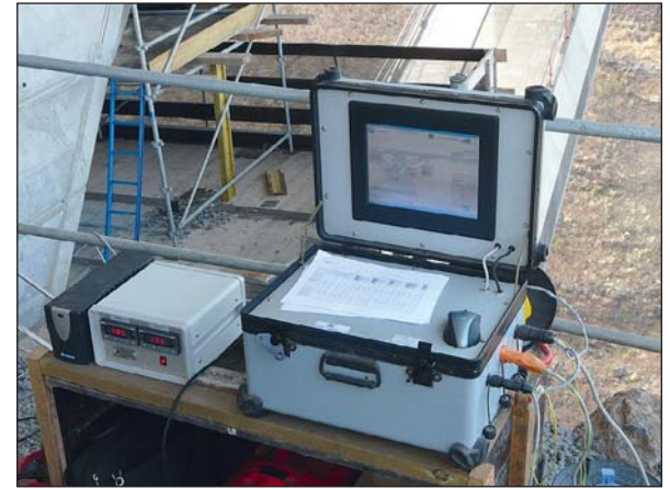
Photo 23 Monitoring de l'instrumentation en phase de construction Instrumentation monitoring during the construction stage
