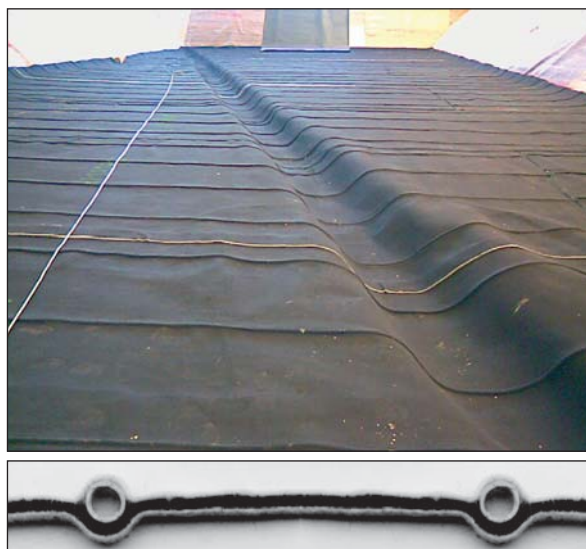
Photo 4 Protection et drainage de la géomembrane Protection and drainage of the geomembrane barrier
