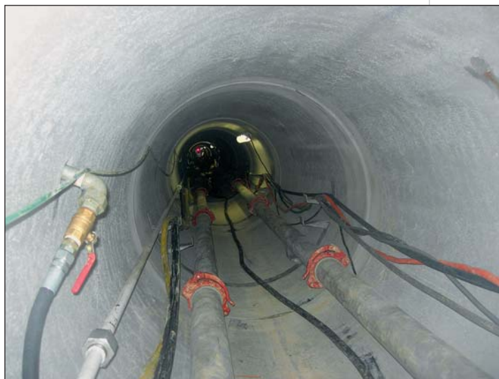
Photo 9 Vanne d'injection Injection valve
