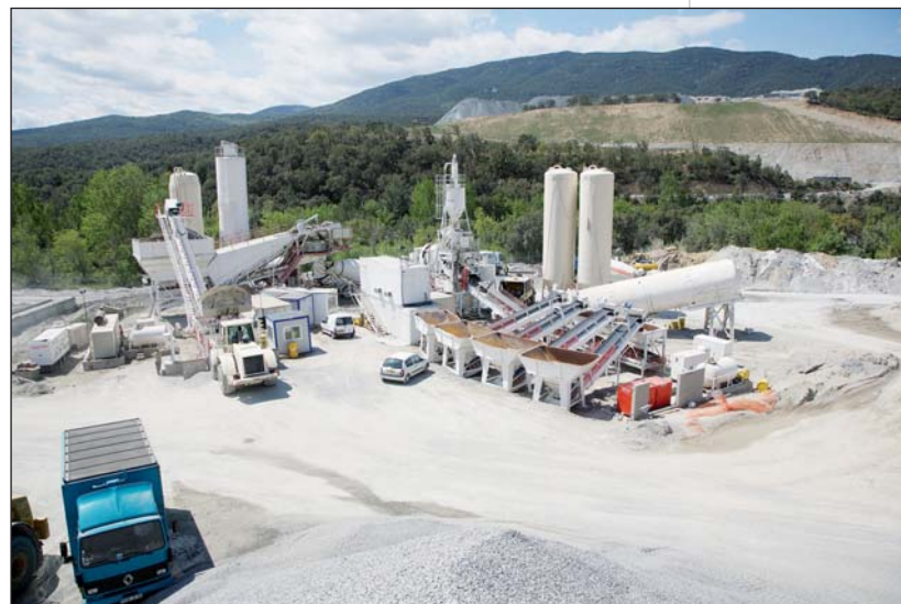
Photo 6 Centrale de fabrication des bétons Concrete mixing plant
