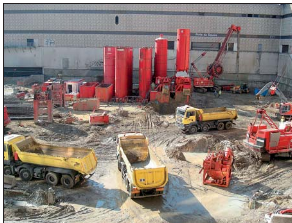
Photo 2 Centrales à boue Slurry mixing plants
