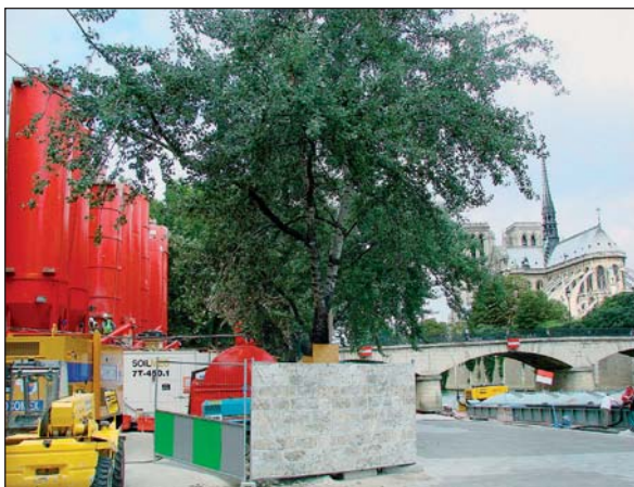
Photo 1 Installation extérieure External installation
