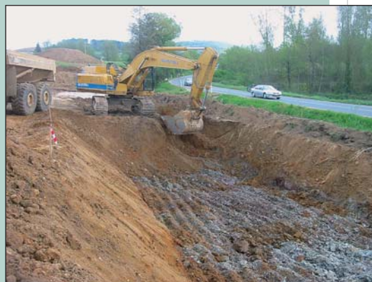
Photo 8 Bêche de pied du remblai R 405 en bordure de la RN 89 Cutoff wall at the base of embankment R405 on the edge of highway RN 89
