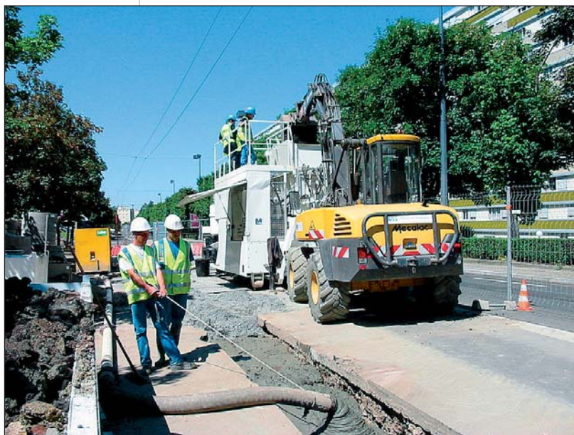
Photo 2 Vue d'ensemble d'un atelier type General view of typical equipment
