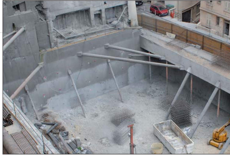
Photo 7 Butons et bracons côté nord Stays and braces on the northern side
