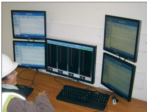
Figure 7 Système GROUT I.T. : poste de contrôle GROUT I.T. Operator during Grouting Operation
