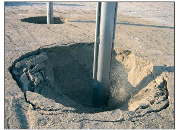
Figure 6 La dimension des cratères formés pendant la vibro- compaction est un indicateur du bon compactage du sol The size of the craters formed during vibrocompaction is an indicator of good soil compaction
