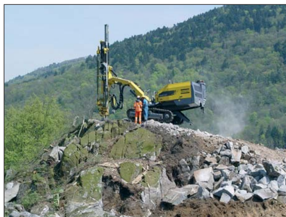
Photo 2 Formation sur foreuse commandée à distance par radio-guidage (Atlas Copco Roc D7 RRC) Training on drilling machine remote controlled by radio guidance (Atlas Copco Roc D7 RRC)
