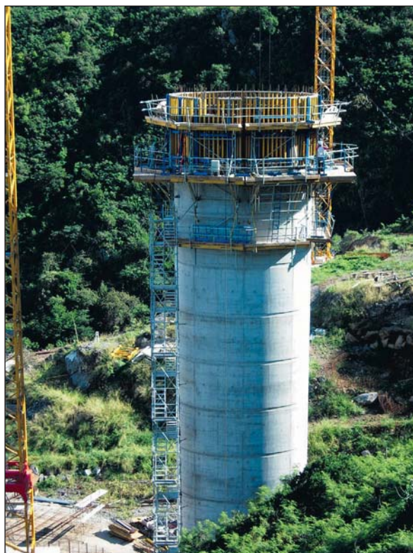
Photo 6 Coffrage des piles P1 et P2 Formwork for piers P1 and P2
