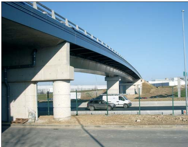
Photo 17 Ouvrage de franchissement de la RN 186 - Aspect final (avant intervention du lot VRD) Bridge over the RN 186 highway - Final appearance (before the main services work section)
