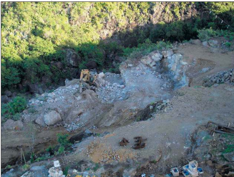
Photo 3 Terrassements de la fouille de la semelle P1 Excavation earthworks for footing P1
