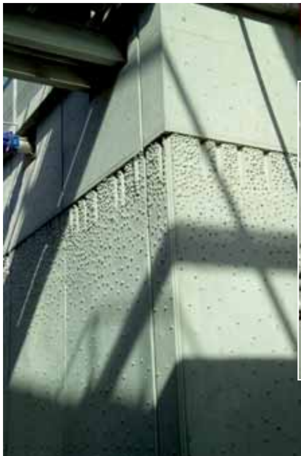
Panneau béton matricé des bassins nitrifiants Matrix concrete panel of the nitrification basins
