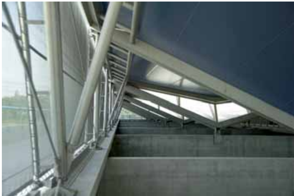
Vue de la charpente métallique support des couvertures des bassins nitrifiants View of the steel structure supporting the nitrification basin covers
