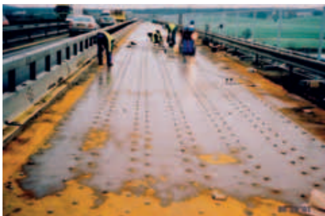
Photo 13 Contre-perçage et pose des boulons HR Counter-drilling and installation of high-strength bolts
