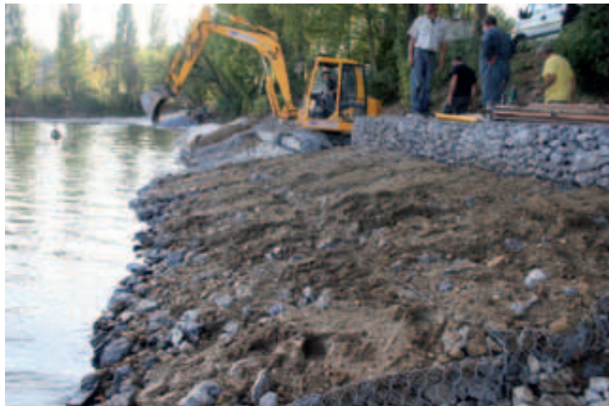
Photo 5 Pose des gabions et matelas de gabions Laying gabions and gabion mattresses
