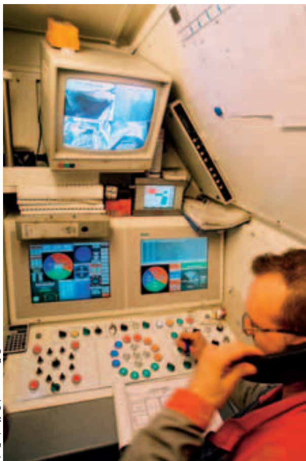
Photo 5 Poste de pilotage Control station
