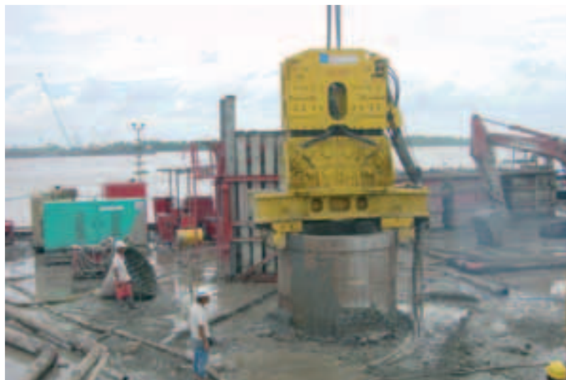
Photo 2 Can Tho - Fonçage de la virole de tête au vibrofonneur Can Tho - Driving the end shell by vibratory driver
