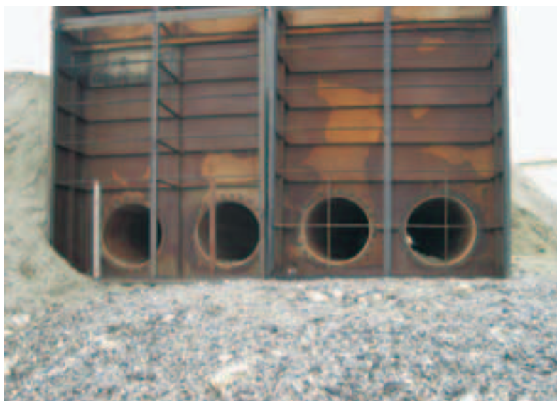
Photo 8 Ensemble de caisses de décantation Set of settling tanks
