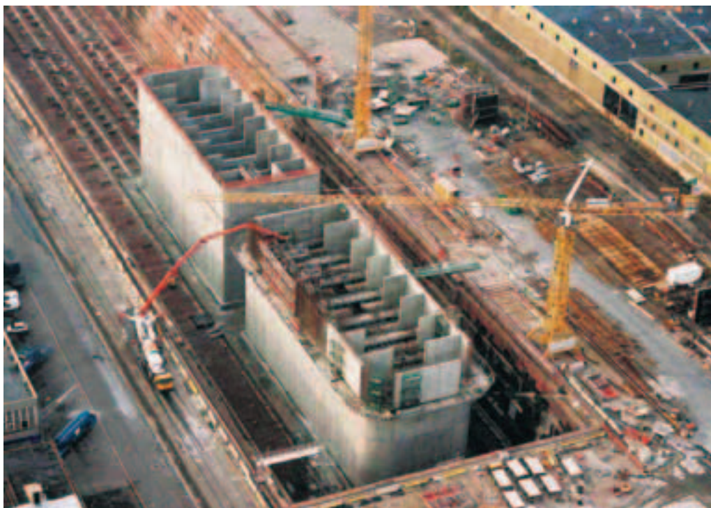
Photo 5 Construction des caissons musoirs en forme 7 Construction of the pier head caissons in dry dock 7
