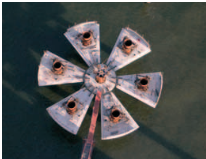
Photo 6 Gabions de protection. Assemblage des "pétales" en béton armé Protective gabions. Assembly of the reinforced concrete "petals"
