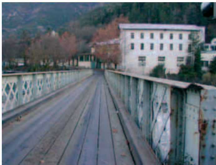
Photo 1 Vue de l'ancien pont sur le Var View of the former bridge over the Var
