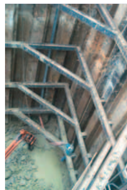
Photo 9 Terrassement du calcaire au brise-roche hydraulique dans le puits "Parking" Earthworks in limestone by hydraulic rock breaker in the "Car park" shaft
