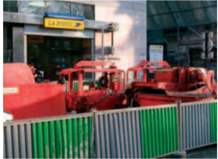
Photo 8 Centrale d'injection rue Lancry à Paris Cement grouting plant in Lancry street in Paris
