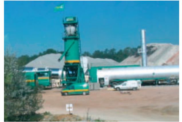
Photo 18 Centrale enrobés Bituminous mixing plant
