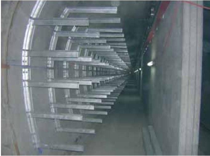
Photo 15 Equipements du tunnel de Kwai Chung Kwai Chung tunnel equipment
