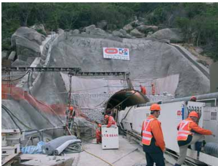
Photo 3 Portail sud du tunnel de Chi Ma Wan et amorce du tunnel South portal of the Chi Ma Wan tunnel and start of the tunnel face
