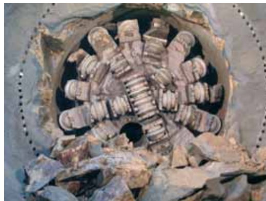
Photo 5 Percement du tunnelier de Chi Ma Wan Drilling by the Chi Ma Wan tunnel boring machine
