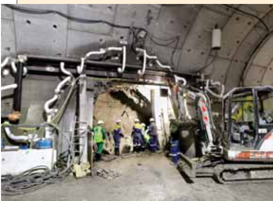
Installations en tunnel Installations in tunnel
