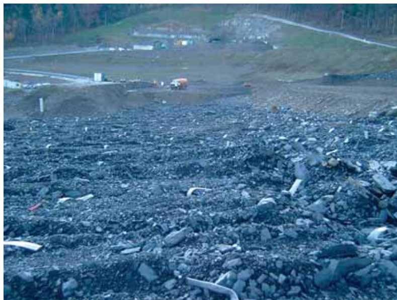
Photo 1 R8 base drainante et drains verticaux R8 draining base and vertical drains
