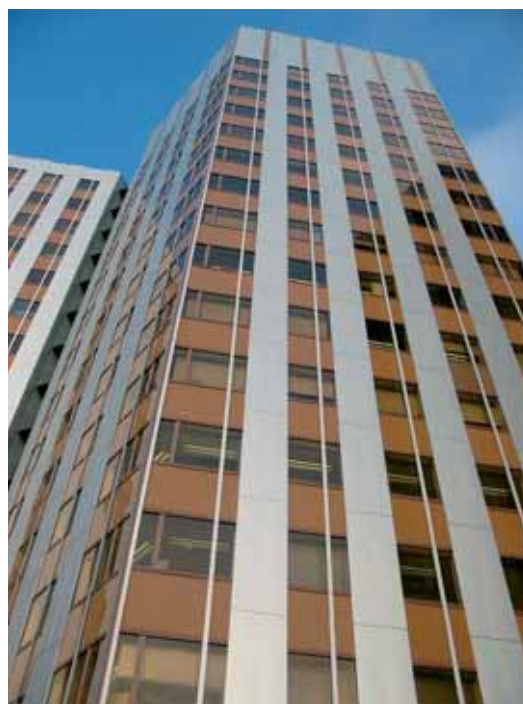
Façades de la tour avant travaux Facades of the building before the works
