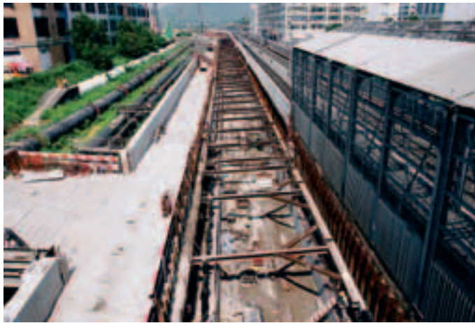
Photo 6 Tranchée Est adjacente aux voies ferrées East trench adjacent to the railway tracks
