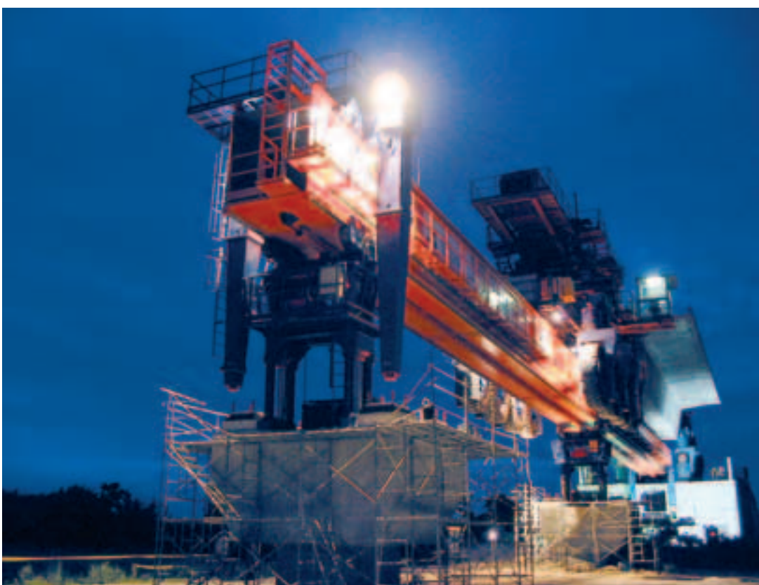
Photo 2 Lancement de la poutre support de nuit Launching the supporting girder by night
