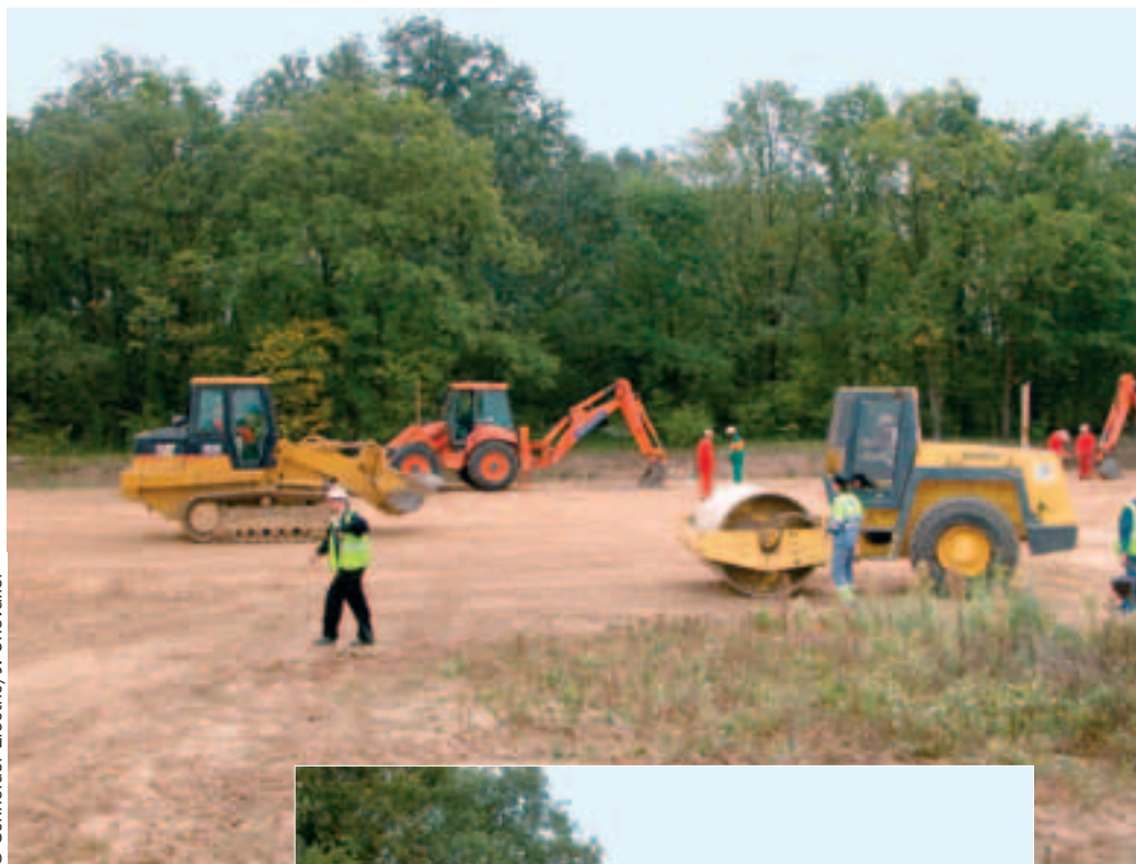
© Schneider Electric/J. Chevallier
