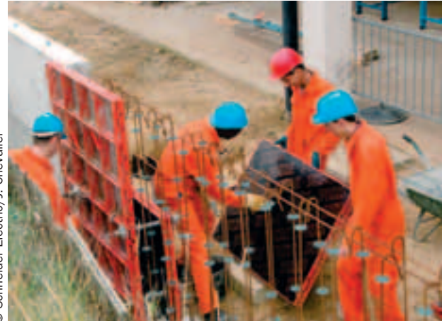
© Schneider Electric/J. Chevallier
