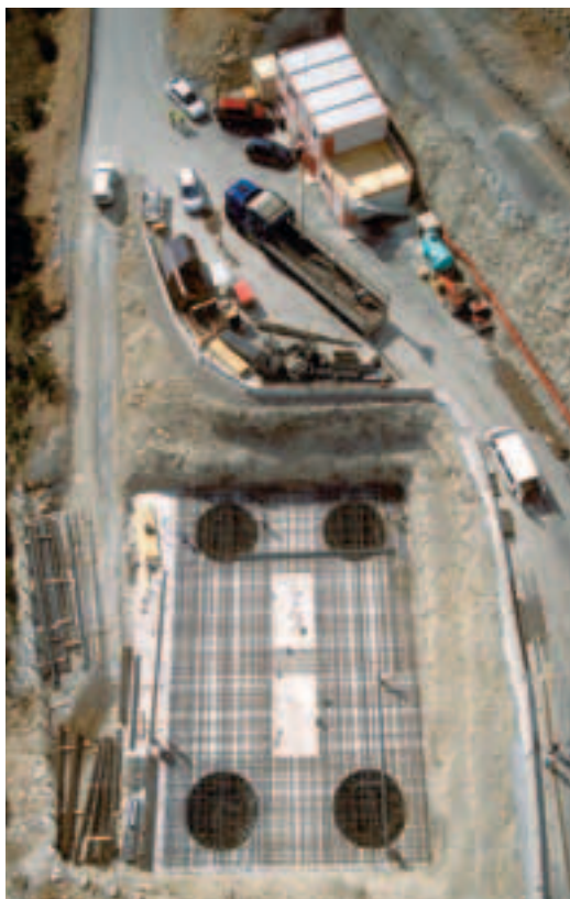
Photo 3 Puits marocains de la pile P2 "Moroccan well" shafts for pier P2
