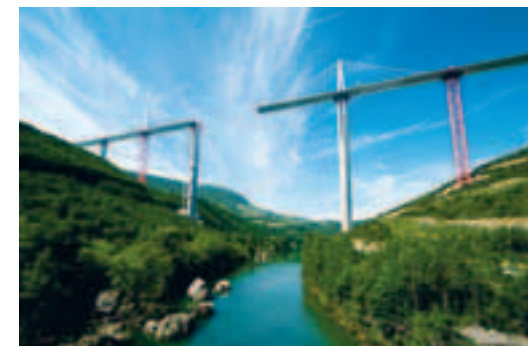
Photo 1 Etat de la structure avant le dernier lançage et le clavage au droit du Tarn Condition of the structure before the final launching operation and keying perpendicular to the Tarn
