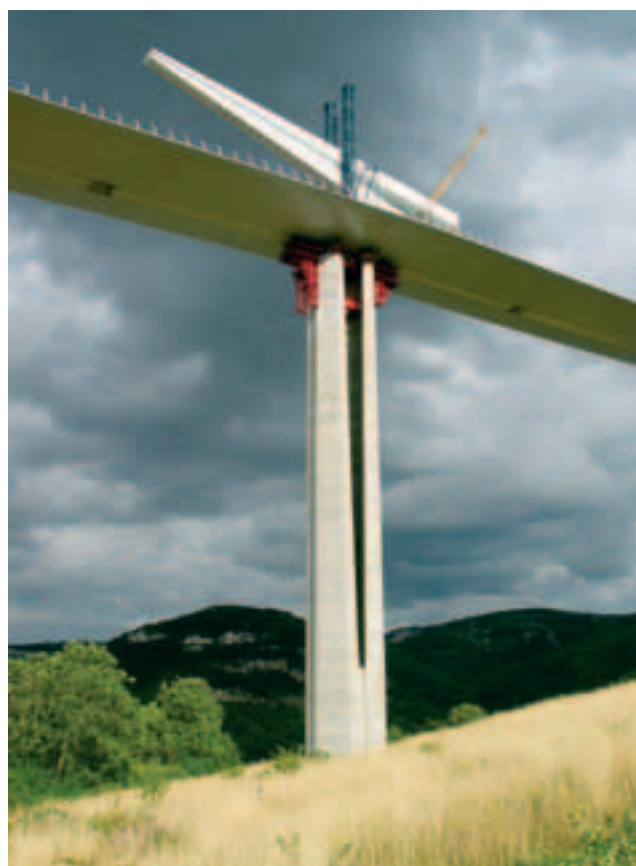
Photo 18 Pylône en cours de relevage sur P1 Tower during raising on P1
