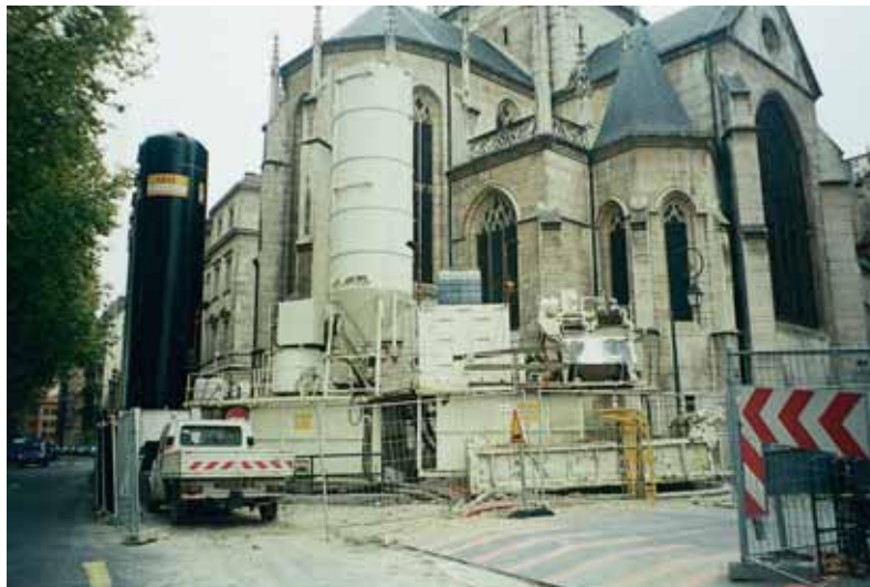
Photo 1 Installation de la centrale à boue Installation of the slurry mixing plant
