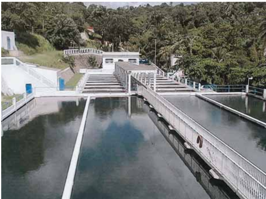
Photo 1 Station de traitement Didier Didier treatment plant
