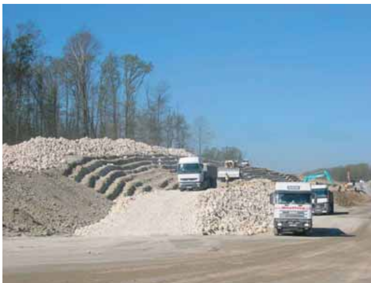
Photo 4 Déblai n° 24533, redans et masque drainant Earth cut No. 24533, keyways and draining facing membrane
