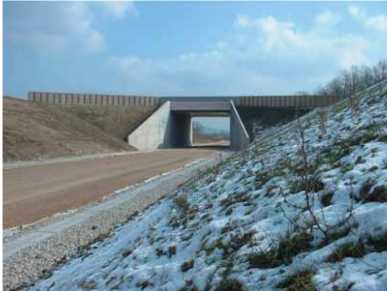
Photo 7 Passage grande faune exceptionnel de 30 m à Villers-en-Argonne Exceptional 30-metre underpass for large game at Villers-en-Argonne
