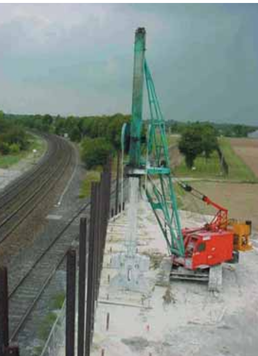
Photo 7 Forage des barrettes pour un pont-rail Drilling supporting wall units for a railway bridge
