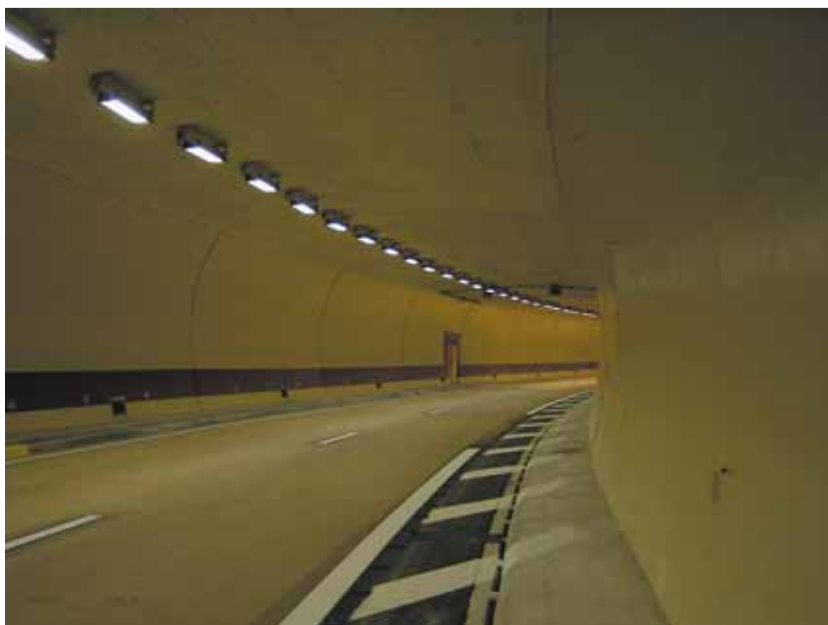
Eclairage en section courante Lighting on link section
