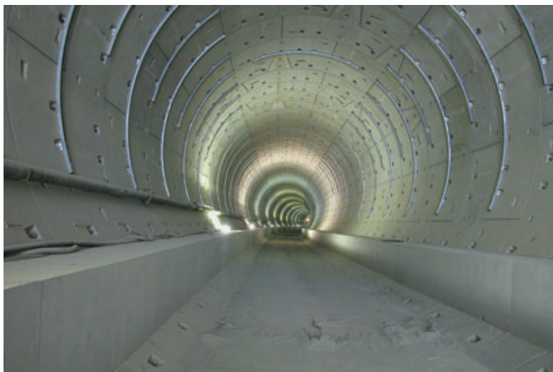
Vue du premier tube en cours d'achèvement View of 1st tunnel tube during the finishing works
