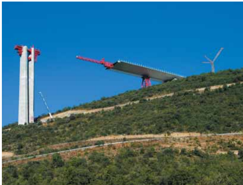
Photo 9 Lançage du tablier côté nord Launching the deck on the north side
