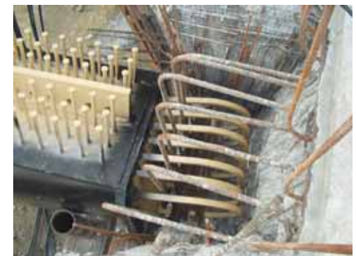
Figure 21 Jonction arc acier - Nervure béton Junction between steel arch and concrete rib
