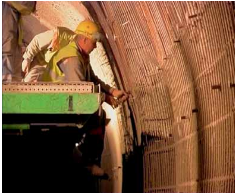
Atelier de pose de treillis soudé Welded wire mesh laying plant
