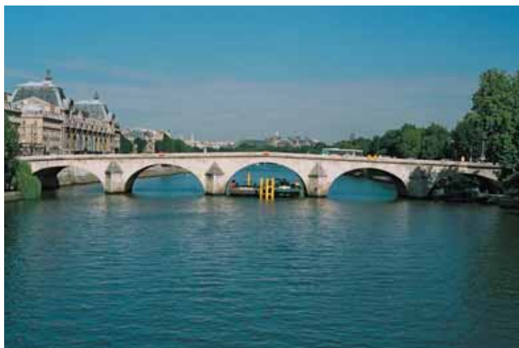
General view of the Pont Royal bridge with its five arches, the "Palais du Louvre" on the left, and the "Grand Palais" in the background on the right
