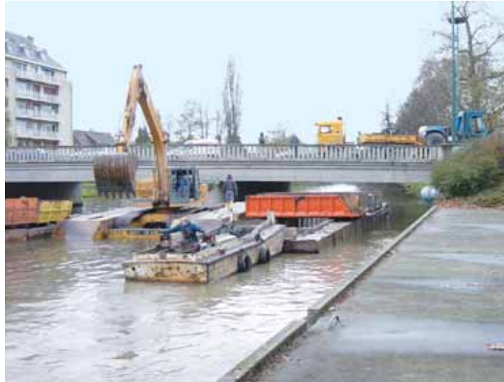
Photo 5 Entre les ponts Bir Hakeim et Churchill, la pelleuse a commencé la destruction des anciens quais Between the Bir Hakeim and Churchill bridges, the power shovel has begun destroying the old quays
