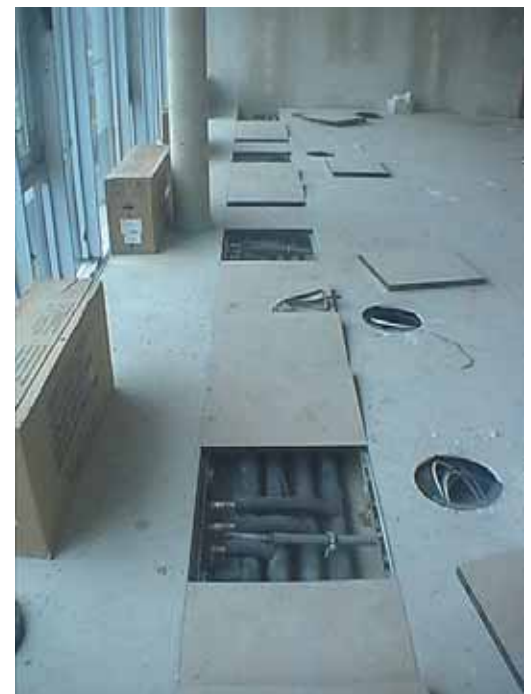
Photo 10 Le faux plancher The raised flooring
