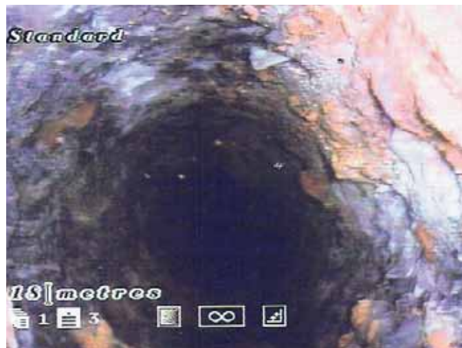
Photo 12 Drain colmaté Clogged drain
