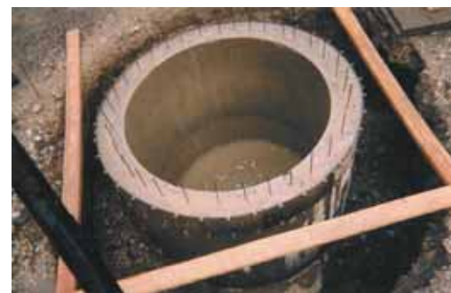
Photo 7 Cuvelage have Cut lining
