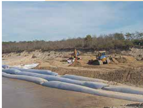
Tubular breakwater on the northern beach during (at top) and after (at bottom) the second storm
