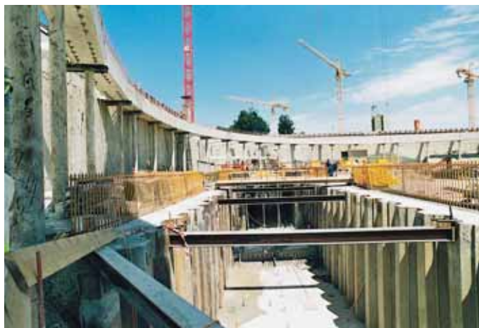
Photo 13 Galeries techniques Main services ducts
