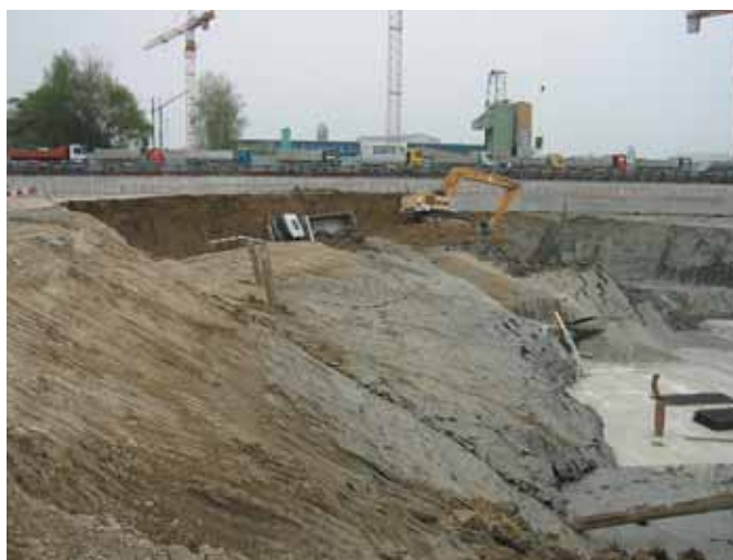
Photo 12 Terrassement - Rupture circulaire Earthworks - Circular break
