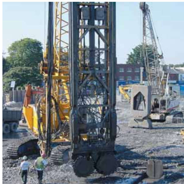
Photo 5 Ateliers Trench Cutter BC30 et benne Trench Cutter BC30 and skip equipment
