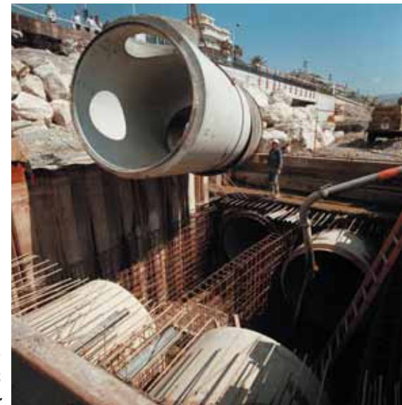
Photo 7 Chambre de raccordement Junction chamber
