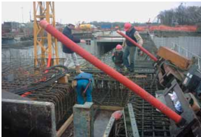
Bétonnage dalle supérieure station Argoulets Concreting the upper slab of Argoulets station
