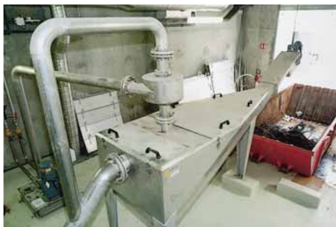
Plant room : grit chamber
