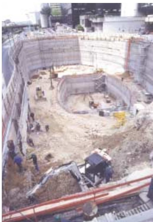
Photo 4 La fouille et les berlinoises The excavation and the Berlin-type retaining walls
