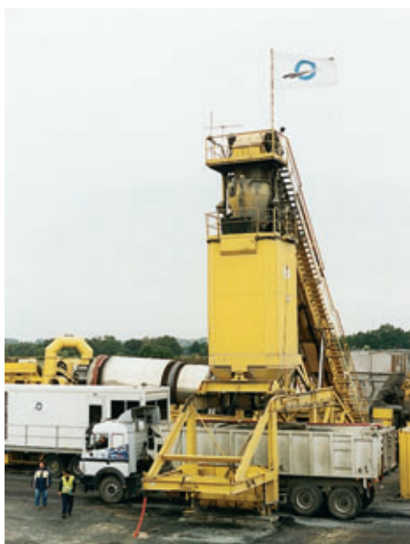
Photo 1 Centrale mobile de fabrication TSM 25 Major Mobile mixing plant : TSM 25 Major
