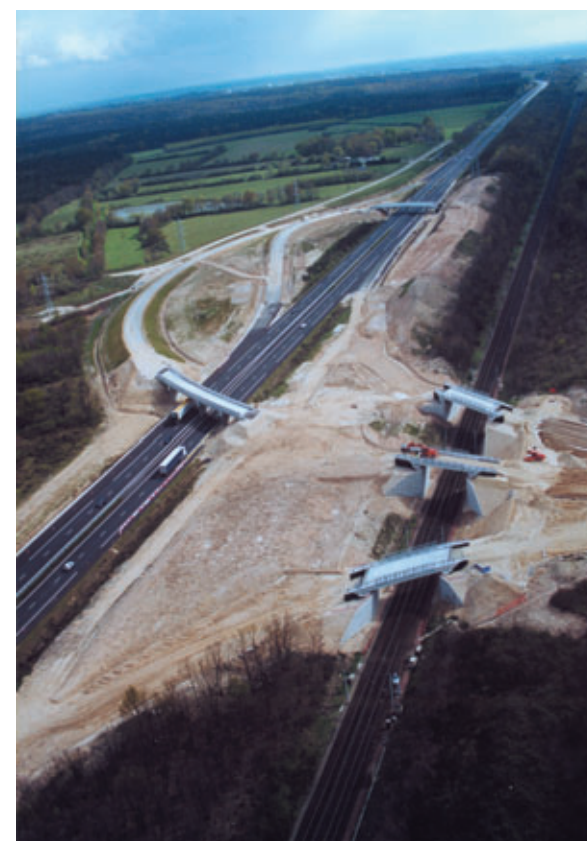
Photo 5 Ouvrages de la bifurcation de Theillay Civil engineering structures for the Theillay junction
