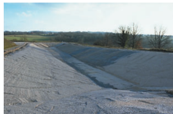
Bassin nu Bare reservoir
