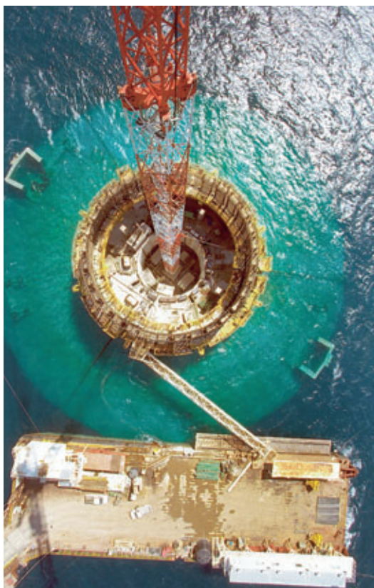
Photo 6 La pile M2 vient d'être installée sur le wet dock The M2 pier has just been installed on the wet dock
