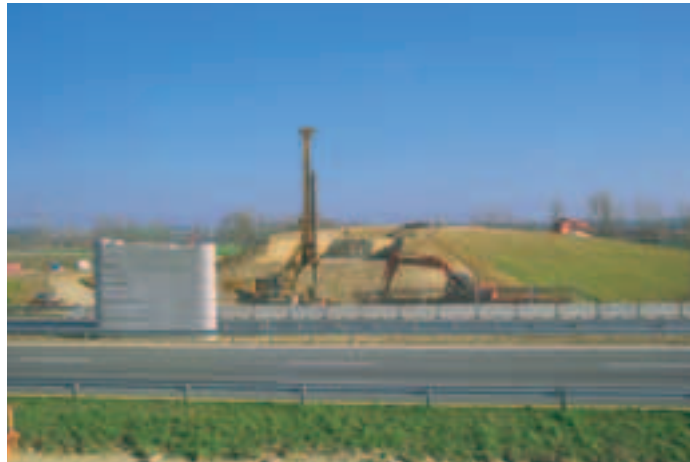
Photo 17 Pile P3 du PS 003 terminée, fondations pile P2 Pier P3 of overpass 003 completed, foundations of pier P2
