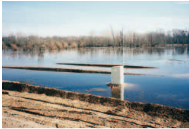
Photo 4 Poste de mesures inondé pendant les travaux Measurement station flooded during the works
