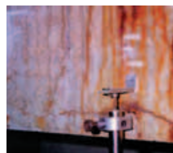
Figure 4 Fissuration du béton d'enrobage Cracking of coating concrete
