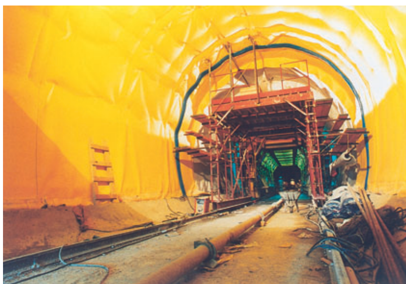
Photo 3 Pose de la membrane en tunnel Placing the membrane in the tunnel
