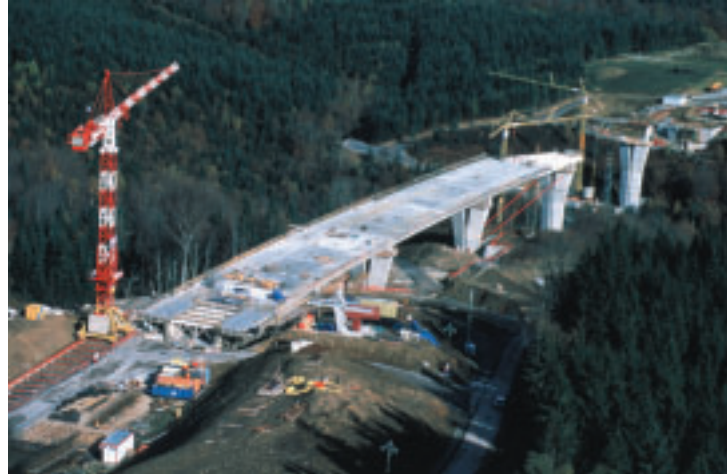
Photos 1 et 2 L'avant-bec accoste la pile, haubanée provisoirement The cutwater nears the pier, with temporary staying
