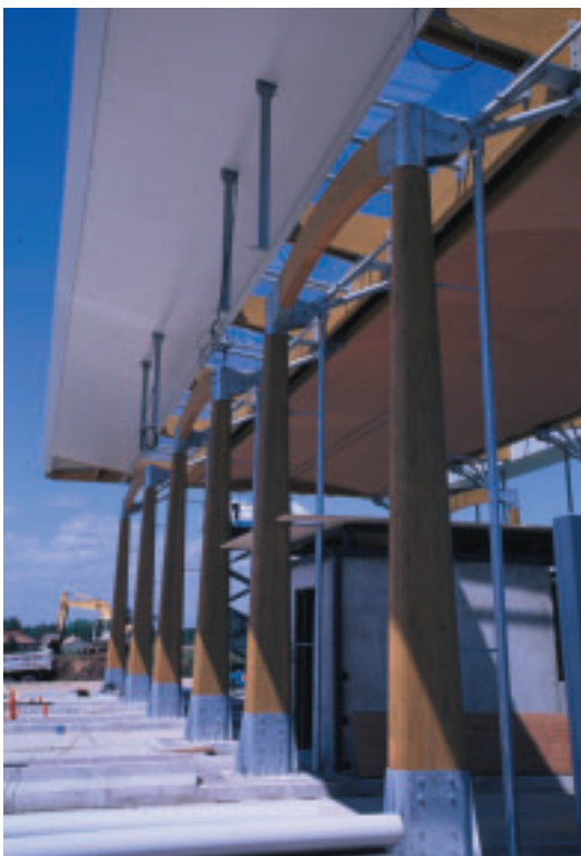
Photo 11 Auvent de la gare de péage de Coutras Canopy of the Coutras toll plaza
