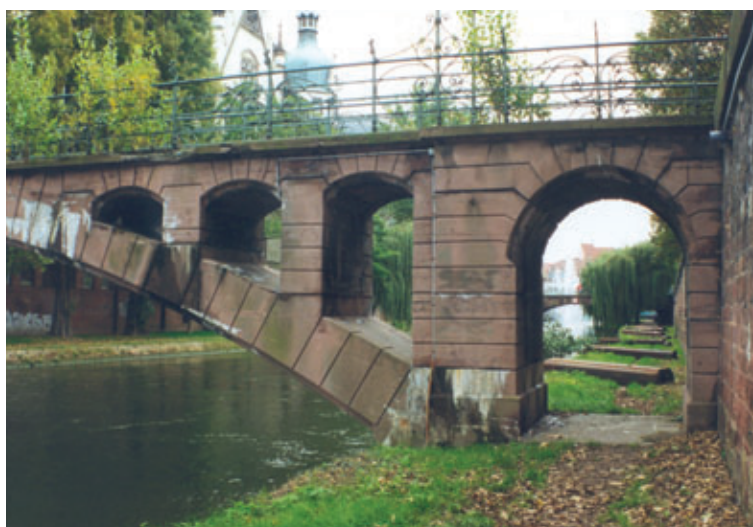
Photo 1 La passerelle existante avant sa démolition The existing footbridge before its demolition
