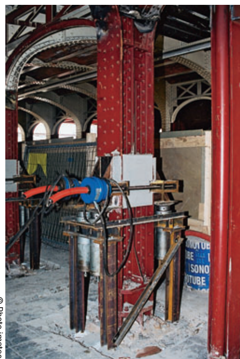
Photo 6 Installation de relevage Hoisting installation
