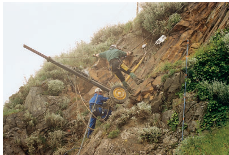
Photo 3 Atelier de forage en station sur zone de clouage Drilling plant in place on nailing zone
