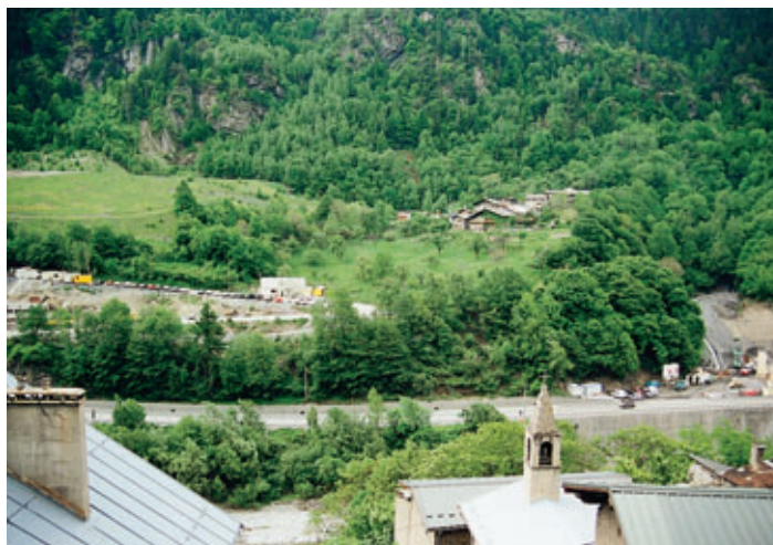
Photo 4 La zone amont de l'éperon avant travaux The upstream zone of the spur before the works
