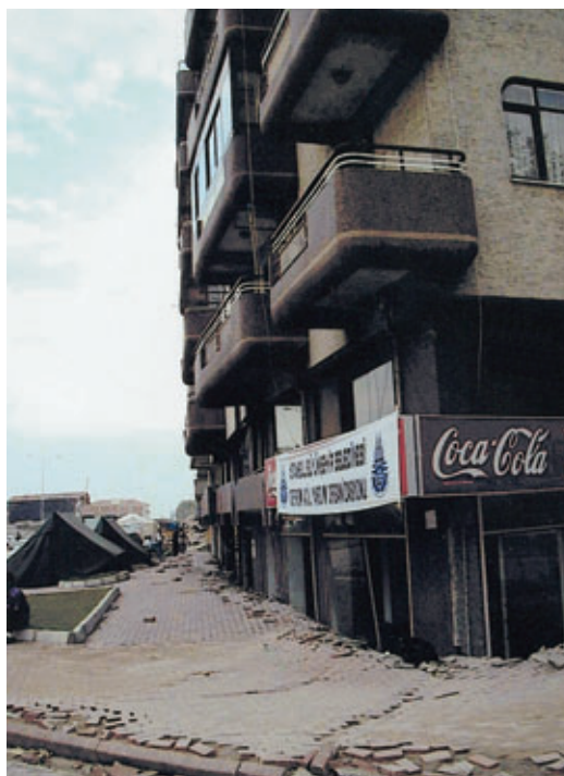
Photo 11 Adapazari - Turquie (1999) : Tassements dus à la liquéfaction de sables lâches Settlements due to liquefaction of unconsolidated sands
