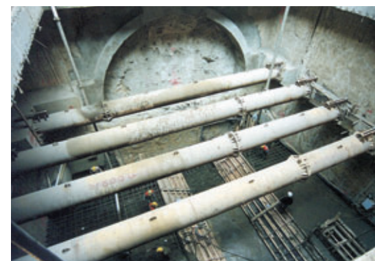
Photo 2 Station excavée et paroi démolie devant le massif de jet grouting du break-out Station excavation and demolished wall in front of jet grouting rock of the break-out
