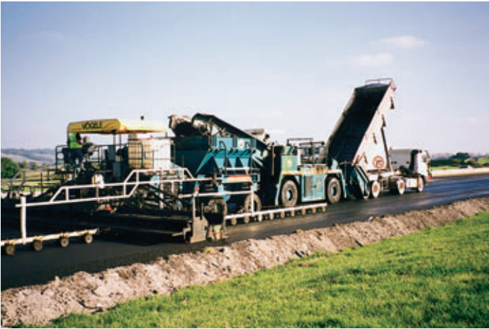
Atelier d'application grande largeur Large-width application plant
