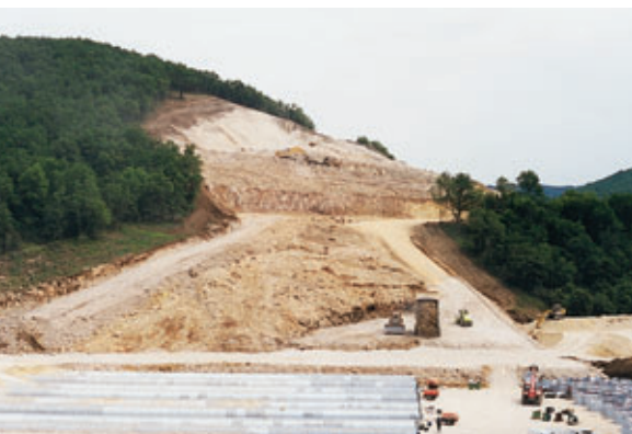
Photo 6 Déblai de Pene et remblai de Loupiac (45 m de dénivellée du terrain naturel) Cut in Pene and fill in Loupiac (45 m difference in level of natural ground sand)
