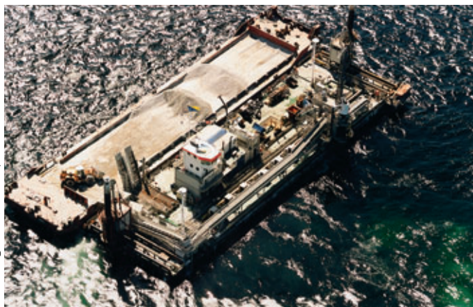
Le ponton multiusage installant le lit de gravier Multi-purpose pontoon installing the gravel bed
