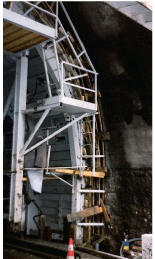
Tunnel head 2. Connection of 70 cm of conventional formwork on the existing head
