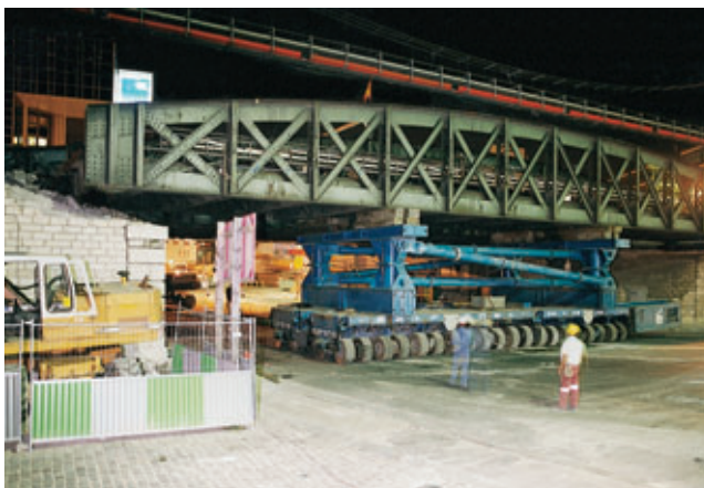
Photo 7 Manutention de l'ancien tablier par chariot "Kamag" Old deck being handled by "Kamag" truck
