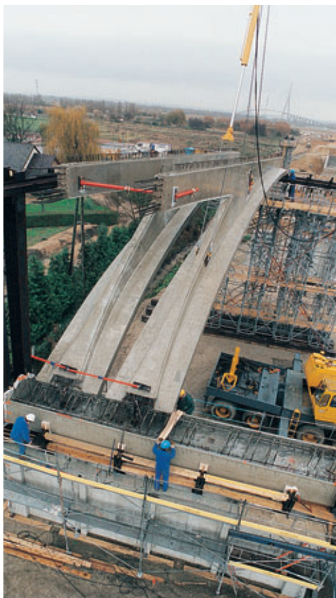
Placing of semi-arches for middle sections, showing the junction at the base of these sections with the shells of the pier heads
